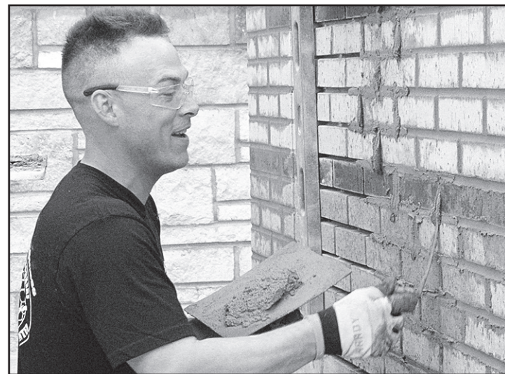
Photo above: Chad Lee, first year Pointer-Cleaner-Caulker apprentice, using a mortar hawk and tuckpointer to tuckpoint mortar joints that have been removed for restoration.
