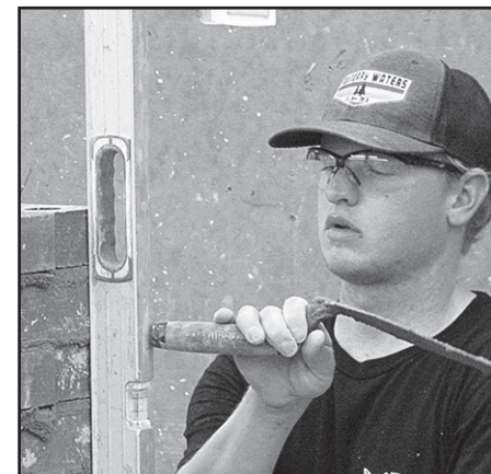
Photo below: Ethan Steen, second year Bricklayer apprentice, using his level to plumb the brick on his project
